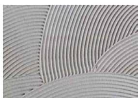
NO Incorrect application
