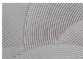
NO Incorrect application
